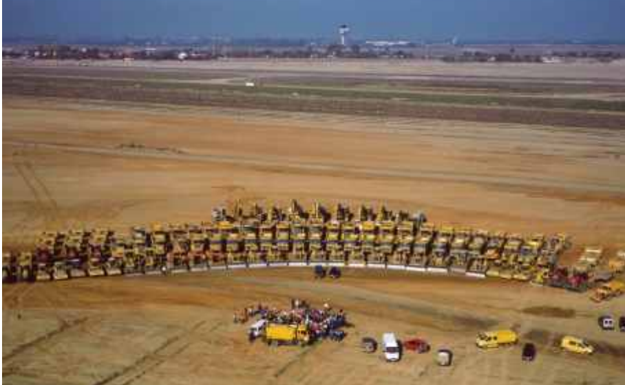
Construction area after a million cubic meters of earth had been moved
