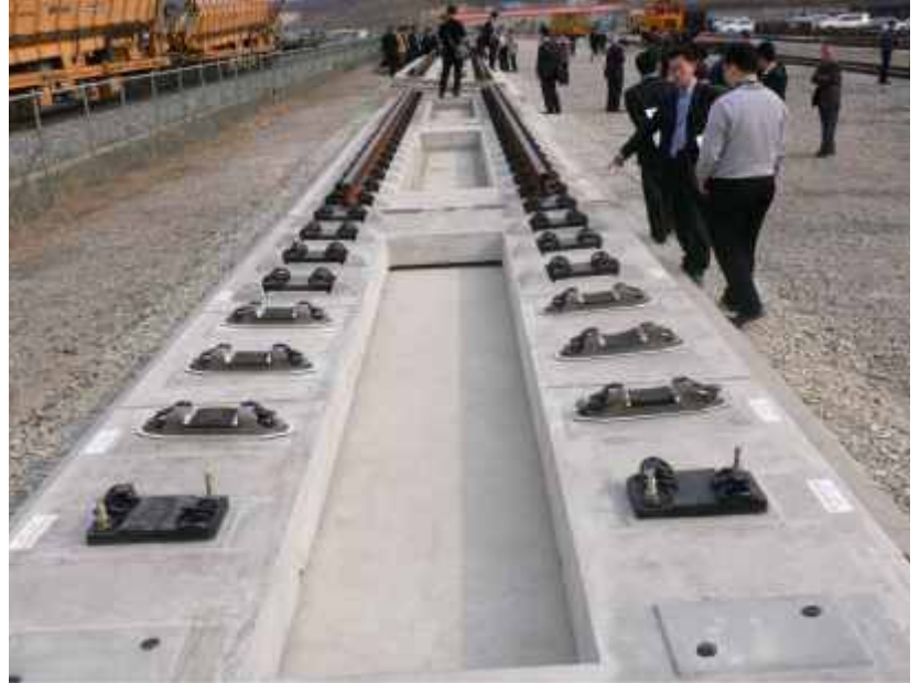
PSTS Frame with a variety of rail supports
